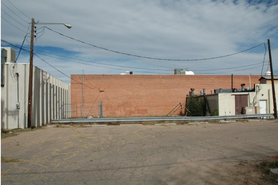
CD 1, Image 67, View to north of south side, and east side of the addition
